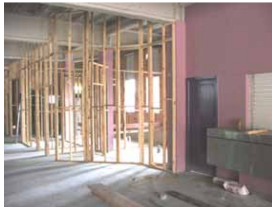
Framework for the new entry and toilets are advancing well at the Kelvin Grove hall.
